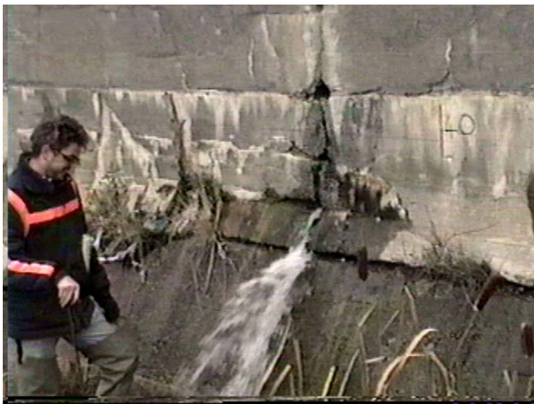
Fuites Seepage (Leaks)
