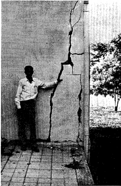
Damage to house in Cuba by swelling soil. The man's left hand is inserted into the crack.
